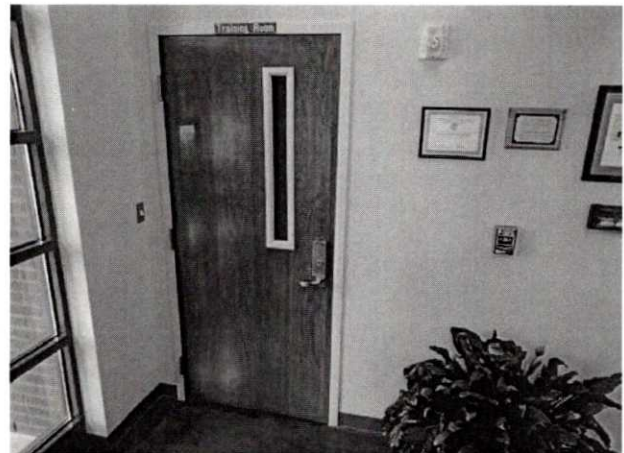
Fire Station #2-Training Room Sign Non-Compliant
