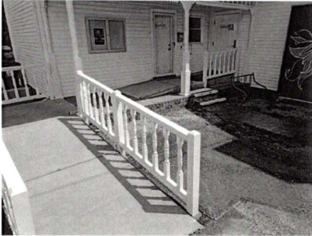
WH Inn Museum-Handrail Non-Compliant
