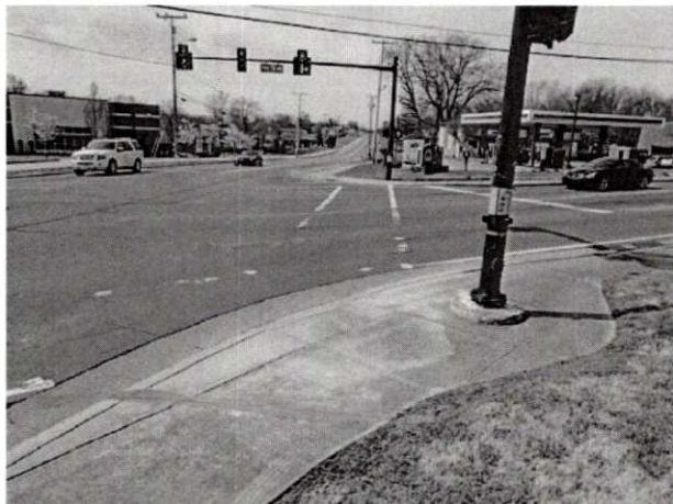
US 31W/SR 76 Crossing 4 Facing 3 (Note Pole in Path)
