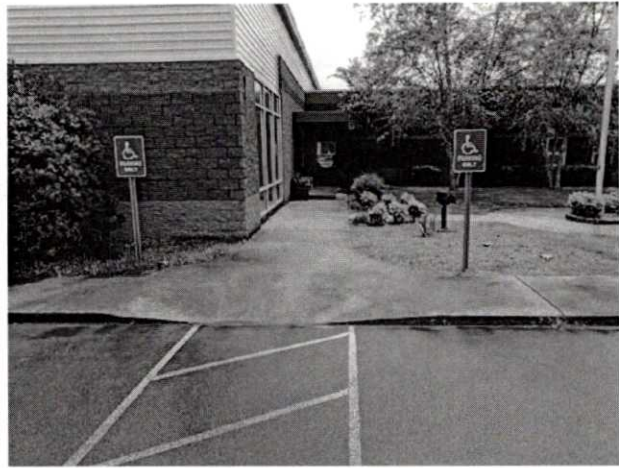
Fire Station #2-No Van Accessible signage (example)
