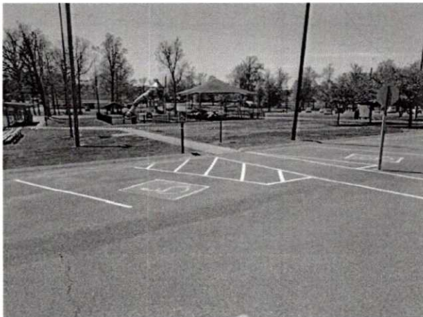
WH Mun. Park-Play Area, Non-Compliant Aisle and Signage
