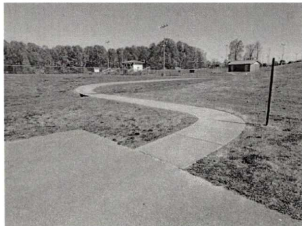
WH Mun. Park-Path to Fields 5 & 6-Exceeds Slope, No Rail over Ditch Crossing, No Path to Bleachers and Fields
