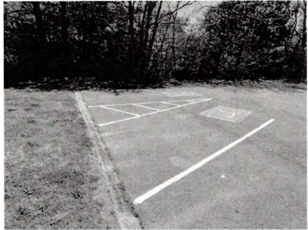
WH Mun. Park- Basketball Court No Signage or Ramp Access
