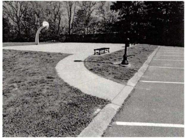
WH Mun. Park BBall Court #1-Non Compliant Ramp
