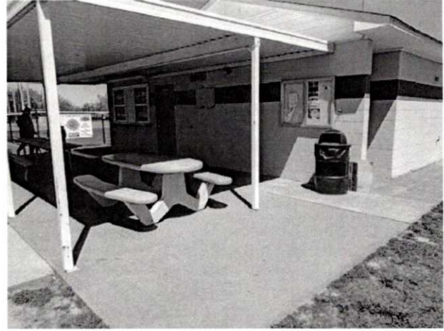
WH Mun. Park Concessions-Table & Window Non-Compliant
