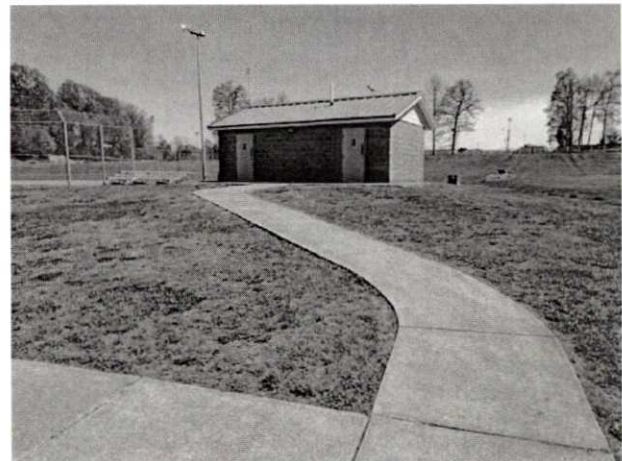
WH Mun. Park-Path to Restrooms Exceeds Slopes
