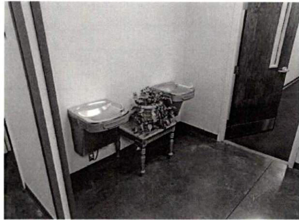
Fire Station #2-Water Fountains Non-Compliant
