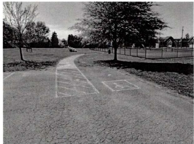
WH Mun. Park-Tennis; No Signage, Faded Paint
