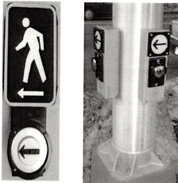
Example of Accessible Pedestrian Pushbuttons
