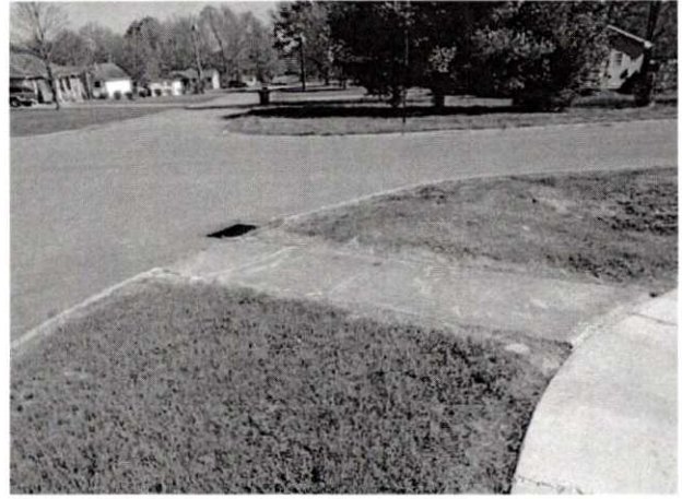
North Wood Park-Ramp Not Compliant
