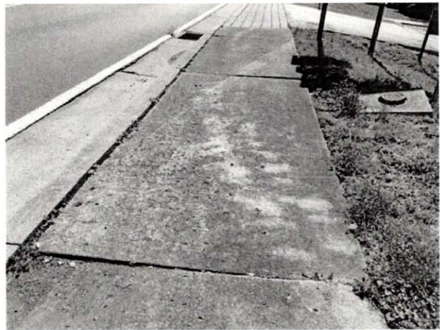
Raymond Hirsch Pkwy-Segment Out of Alignment
