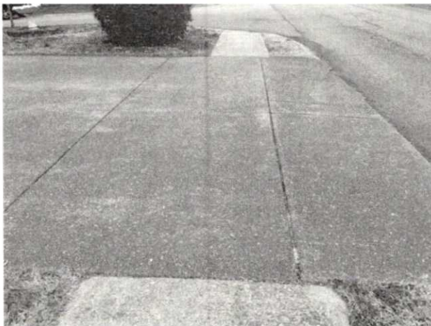
Apache Trail-Typical Driveway Expansion Joint Discontinuity
