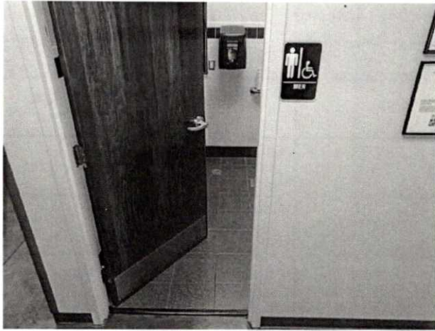
Fire Station #2-Restroom Door Not Self-Closing
