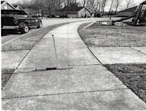
Foster Drive-Example Non-Compliant Cross Slope
