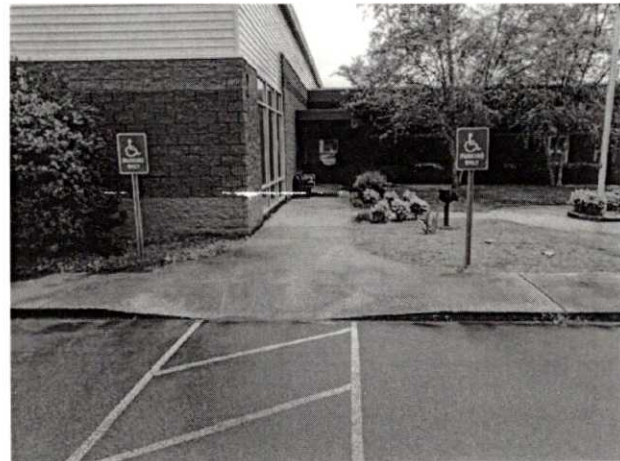
Police Department-No Ramp Detectable Surface Warning
