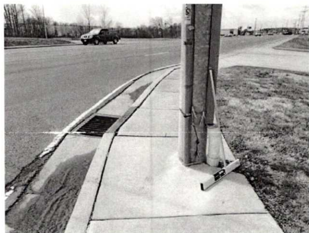
SR 76/Lone Oak-Utility Pole Obstruction
