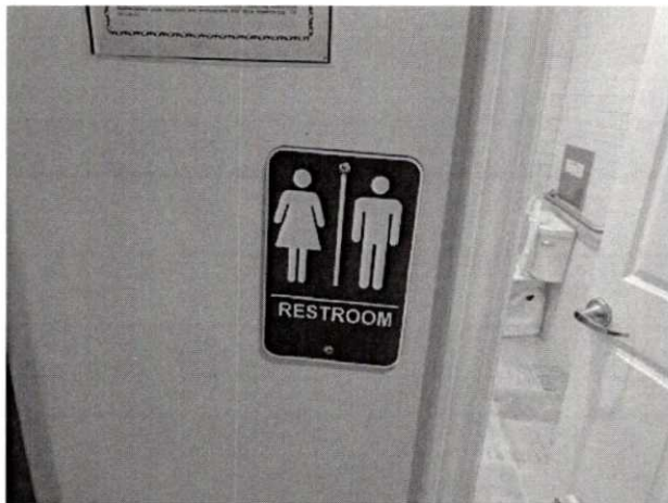
WH Inn Museum-Restroom Sign Non-Compliant
