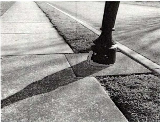
Sundance Way-Light Pole Base Discontinuity
