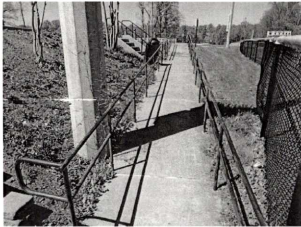
WH Mun. Park-Ramp to Field #7 Exceeds Slope/Length
