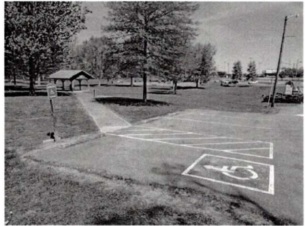
WH Mun. Park-Ramp to Pavilion #1, No Detectable Warning
