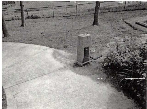
Veterans Memorial Trailhead-Non Compliant Fountain
