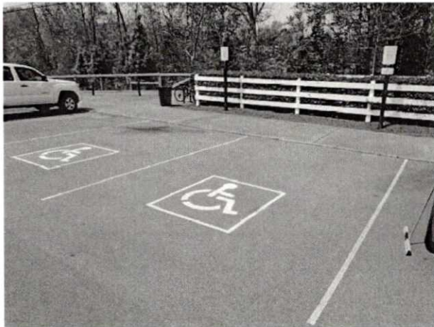
Tyree Springs Trailhead-No accessible Aisle or Ramp
