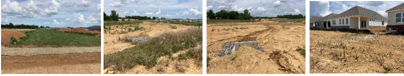
080422008 - Construction EP&SC Inspection: Marlin Pointe: Inspection of the site for failures and adequate controls installed per plans.
