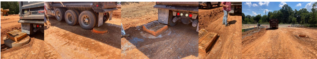
081722009 – Construction Site EPSC Inspection: Springbrook Phase 3&4: Inspection of perimeter controls along buffer.
