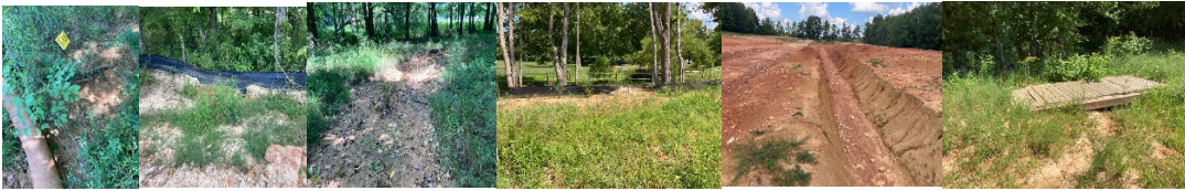
081822004 – Proof Roll: Willow Grove Phase 1: 1 st Lift of Base Stone: Inspection of compaction with a scaled load.
