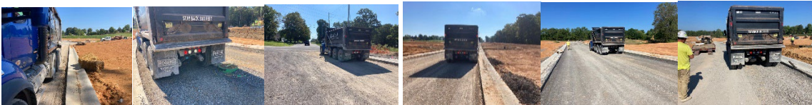
081822005 – Open Trench: Sage Road Development: Infrastructure Inspection of 30”&24” HDPE at F.1 to F.2, F.2 to F.3(F.3 not installed)
