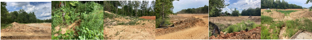
080922002 – Construction EP&SC Inspection: Copes Crossing: Inspection of the site for failures and adequate controls installed per plans.
